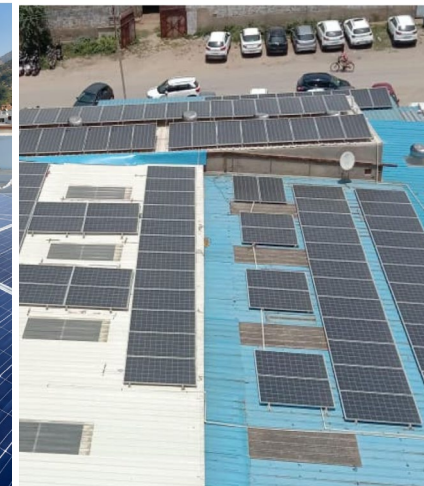
Shivam Hyundai, Ajmer, Rajasthan (50 kWp 2020)
