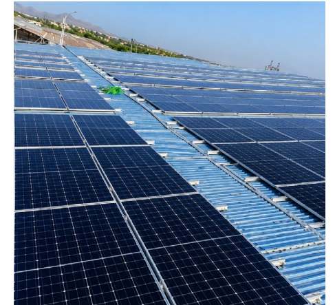
Gayatri Minerals, Rajasthan , (150 kWp 2021)
